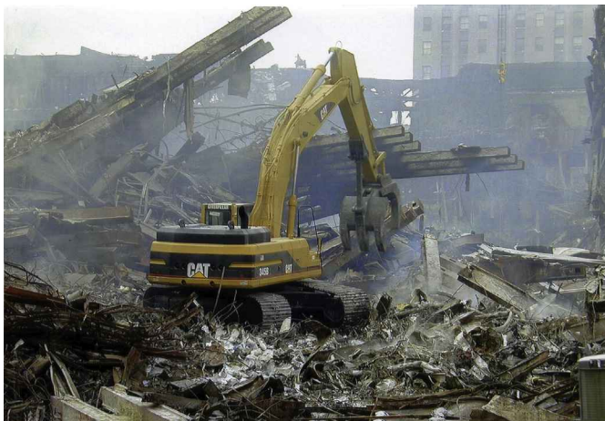
FIGURE 2.2 The Ground Zero Pile. A Caterpillar excavator clears steel and concrete from the wreckage of Manhattan's World Trade Center complex following an attack by hijacked commercial airliners on September 11, 2001.
